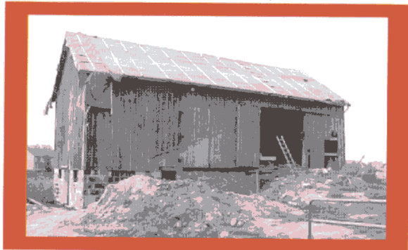
H.A. Hinz Co. began restoration of the barn in the summer of 2005.
